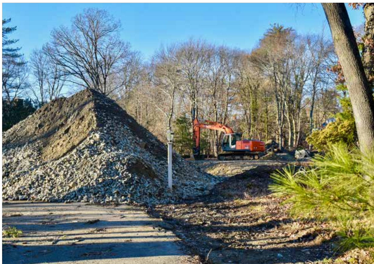
Work begins on a new house on Canton Ave. (Photos by Elaine Cushman Carroll)
